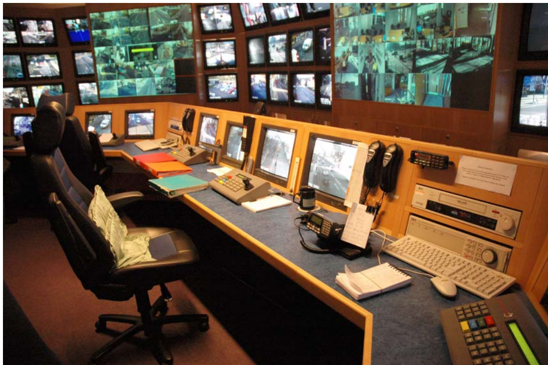
Fig 6: Photograph of the London Borough of Harrow's CCTV control room
